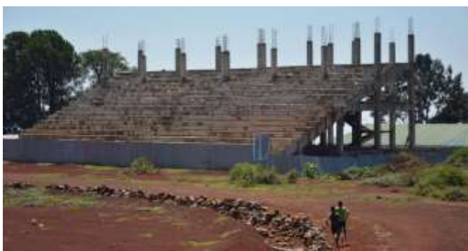
Picture 2: The incomplete Kamariny stadium in Kenya. Photo courtesy of Uroš Kovač
